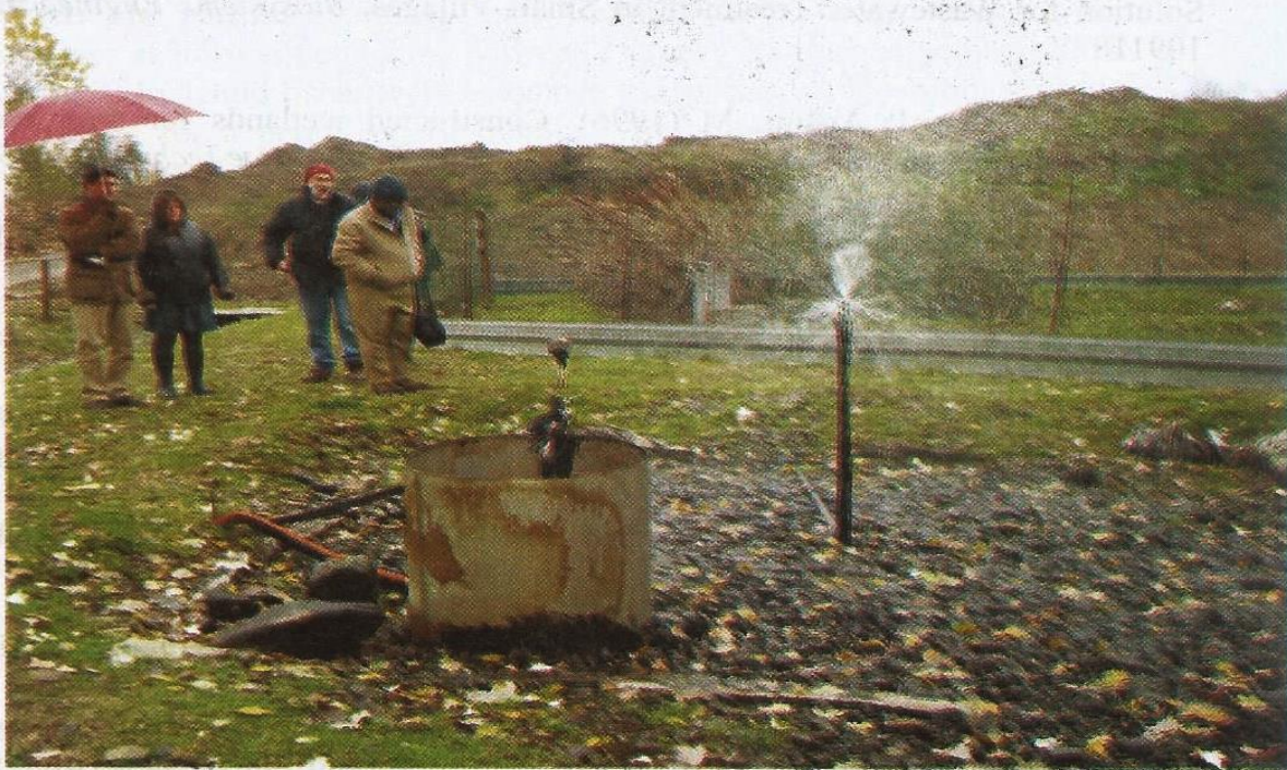
Fig. 10: The last stage of the Phytodepuration system at Bologna showing treated water being sprayed onto an engineered filter bed with biofilm
