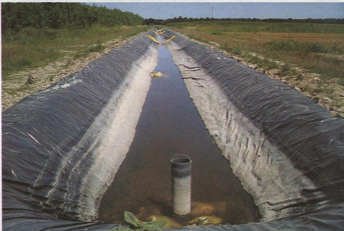
Fig. 7: An impermeable geotextile liner at the bottom of each bed to prevent groundwater contamination
