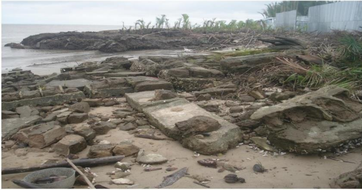
Figure 6: Debris of brick building destroyed by sea level rise in Ibaka, Mbo LGA, Akwa Ibom State (Culled from Umoh et al , 2013)
